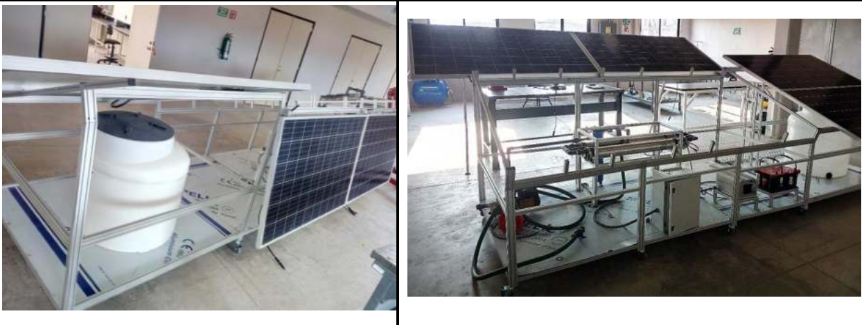
Figure 35.- Stand-alone PV installation on the water potabilizer structure
